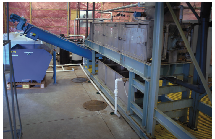
Class A Septage Dewatering Skid Big Fish Environmental Charlevoix, MI
